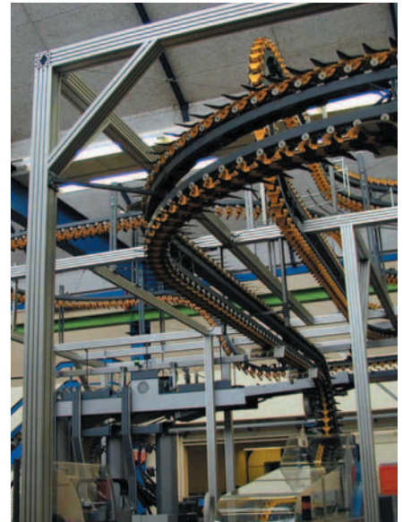
Newspaper handling system
